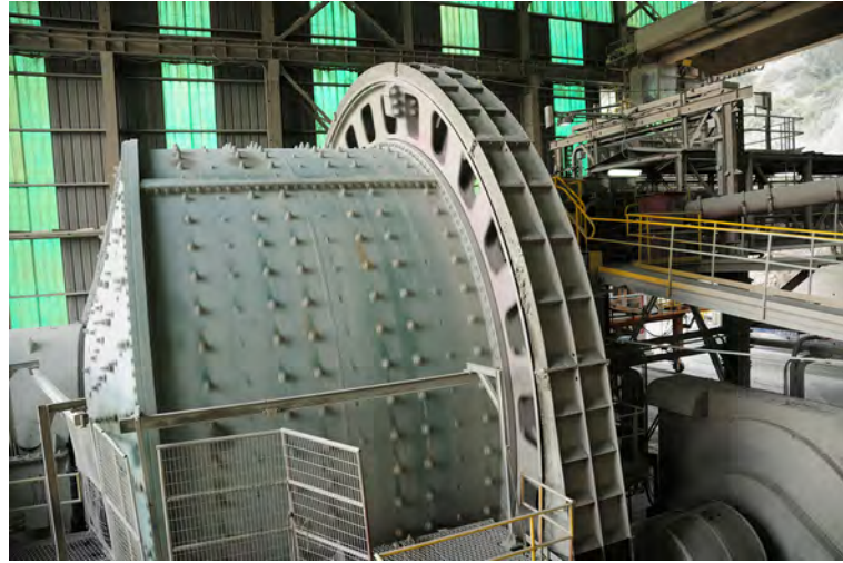
Figure 12: Any induction motor driving a large load such as the ball mill shown above requires a substantial amount of reactive power to operate. Using distributed power factor correction prevents the large reactive power requirement of the motor from affecting the power factor of the industrial application.
